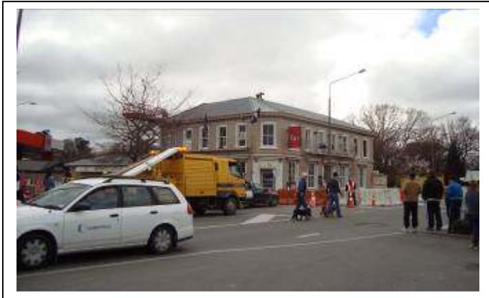
The Famous Grouse Lincoln pub after the earthquake. The roofing is just being removed
